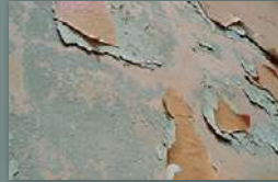
Peeling & Flaking of paint
